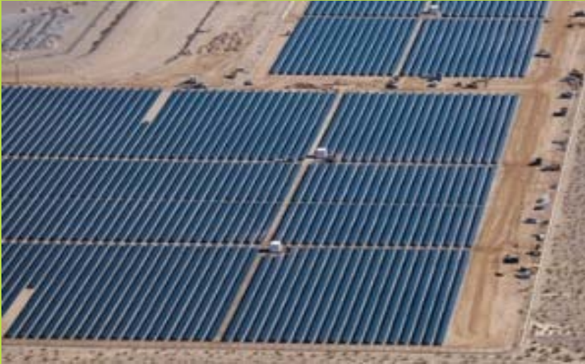
U.S. First Solar, Nevada, (300MW)
